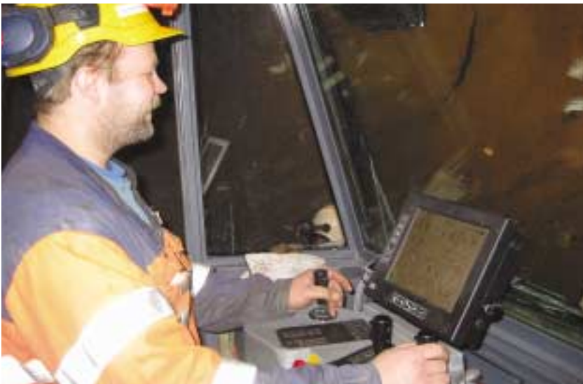
The cabin and the computer control system with double joystick operation helps the operator to achieve high productivity.
