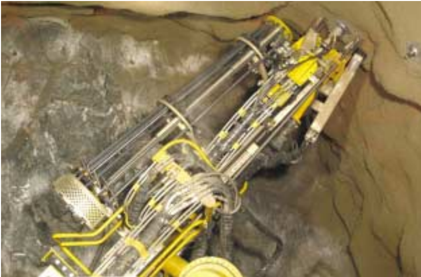
With the Boltec LC and Swellex Mn12 rockbolts operators at Kemi mine are installing some 80-90 bolts per shift.
