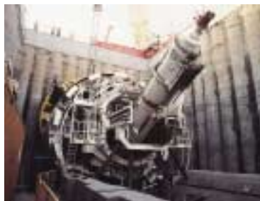
View of the screw conveyor
