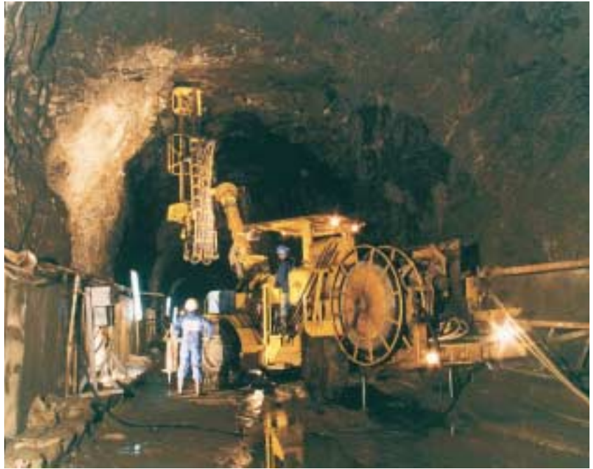
Atlas Copco Boltec 435 H at work in C-1 at Tala Hydro project.
