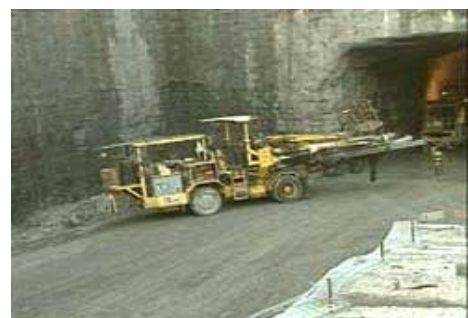
Picture 3: Work under way at the metro extension to Laval in Montreal.
