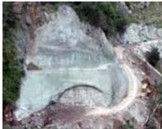
Picture 1: One of the plugged portal on one of the tunnel between Faial and Santana.
