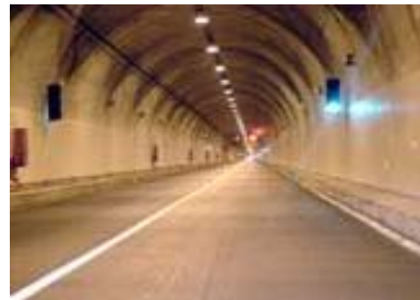
Picture 4: New surfacing needed for the Encumeada tunnel.
